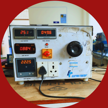
Electrical Test Panel
